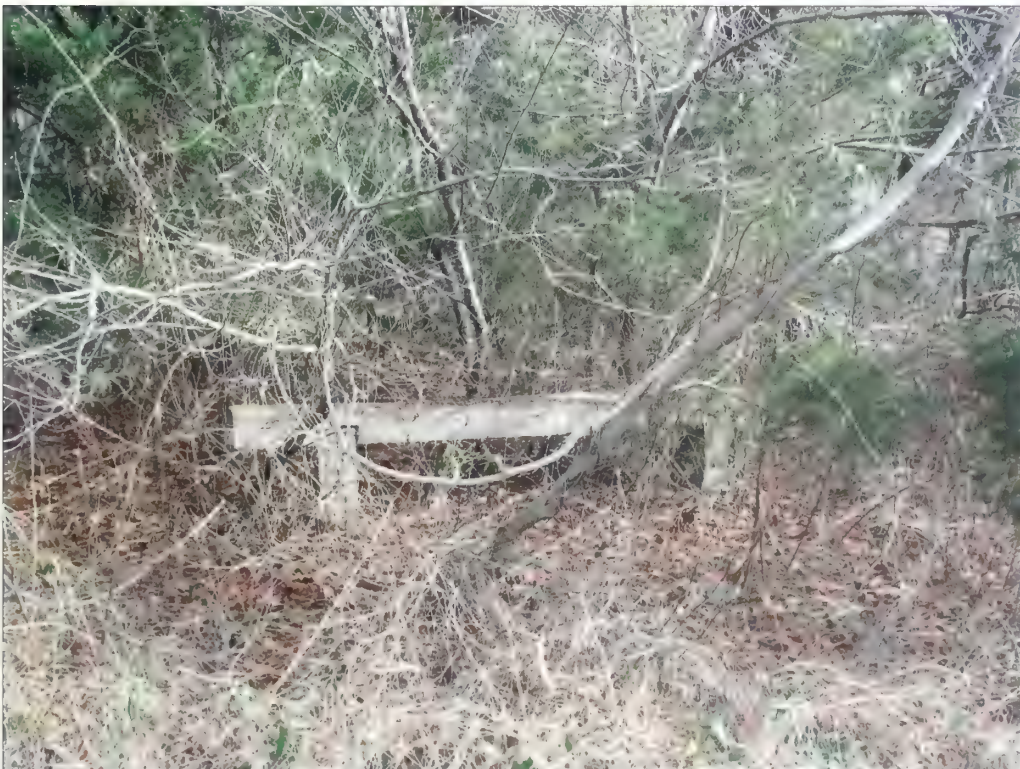
Figure 3.58. View looking east at wood guardrail, Battery Mills. Two series of wood guardrails are installed along the eastern edge of the unpaved road. The guardrails are in fair to poor condition and located across from the gun emplacements (Olmsted Center, January 2009).
